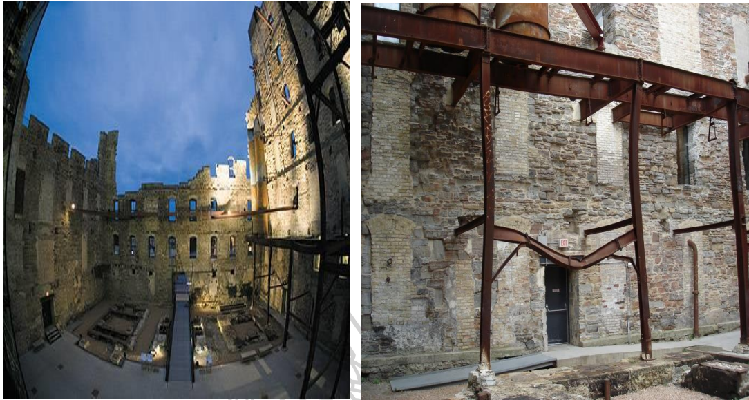
Figure 21 Old Structure Section damaged in a Fire Incident, Retained for Narrating the Place Story
