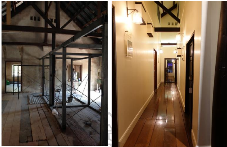
Figure 82 Baan Luang Rajmaitri, Before and After Renovation Source: www.baanluangrajamaitri.com and Researcher, October 2019
