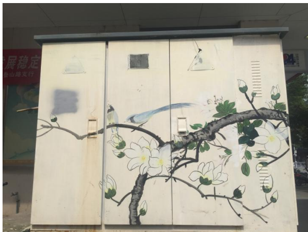
Figure 46 Electric control box installed on the street, the paintings on the surface of the box are created by the artist.
