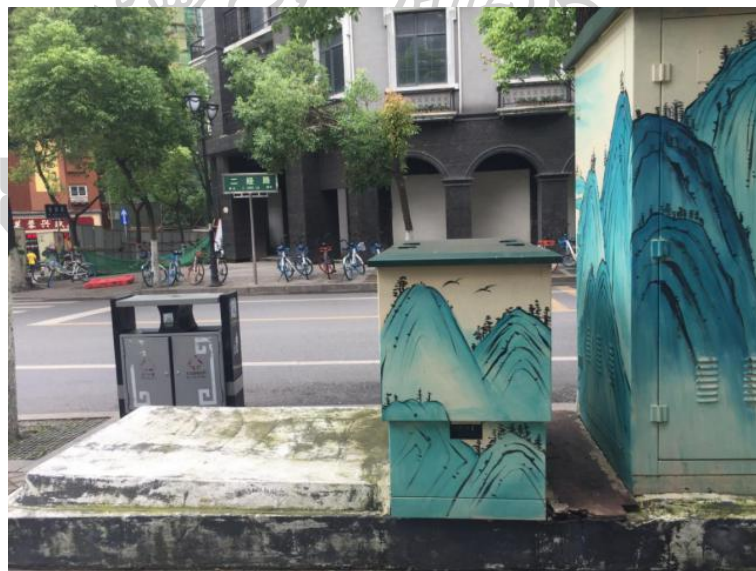
Figure 49 Electric control box installed on the street, the paintings on the surface of the box are created by the artist.
