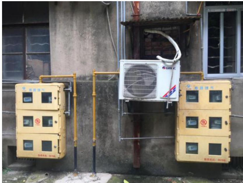
Figure 50 Electrical control box hanging on the wall. Source: Shot by the author in Nanchang, China, March 2019.
