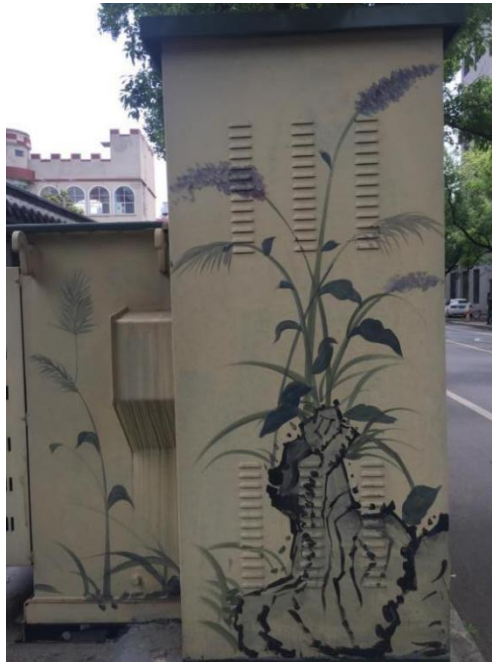
Figure 48 Electric control box installed on the street, the paintings on the surface of the box are created by the artist.
