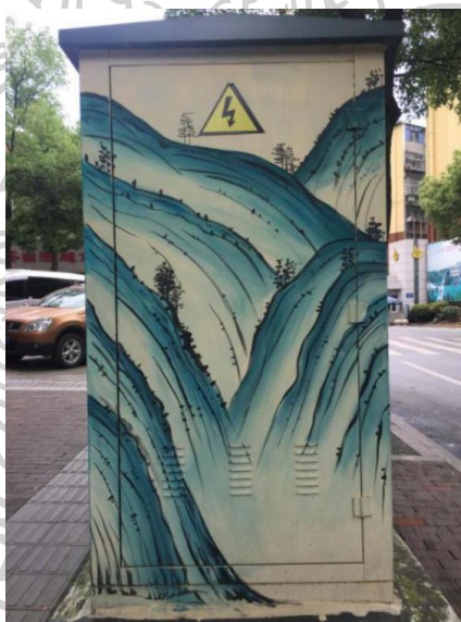
Figure 47 Electric control box installed on the street, the paintings on the surface of the box are created by the artist.
