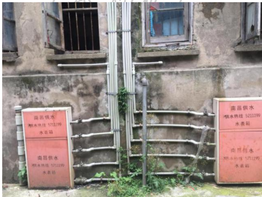
Figure 51 Water meter box hanging on the wall. Source: Shot by the author in Nanchang, China, March 2019.
