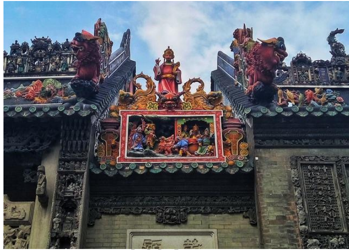
Figure 33 Roofs in southern China are complicated in form and made in detail. With narrative sculpture, it is highly ornamental. (long-focus) Source: Shot by the author in Guangzhou, China, March 2018.
