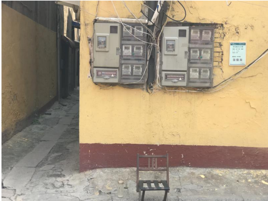
Figure 52 Electrical control box hanging on the wall. Source: Shot by the author in Nanchang, China, March 2019.
