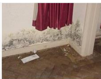
Black mould on wall
