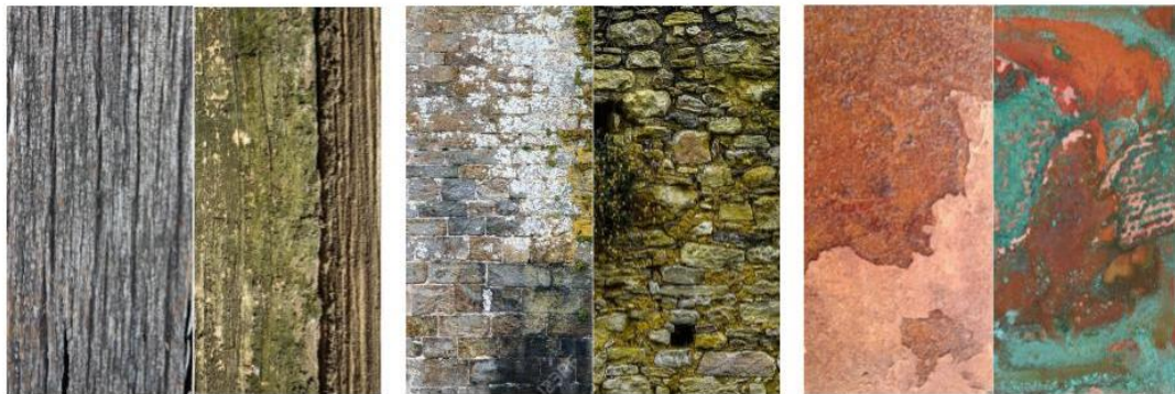
Decayed Wood Skin
