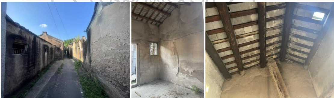
Figure 121. Slightly Damaged Buildings, Woshicun
