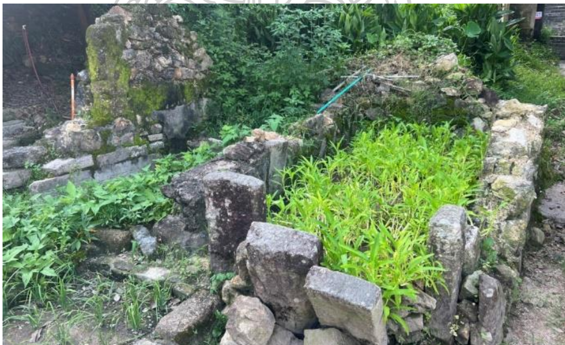
Figure 50. Completely Damaged, Woshicun
