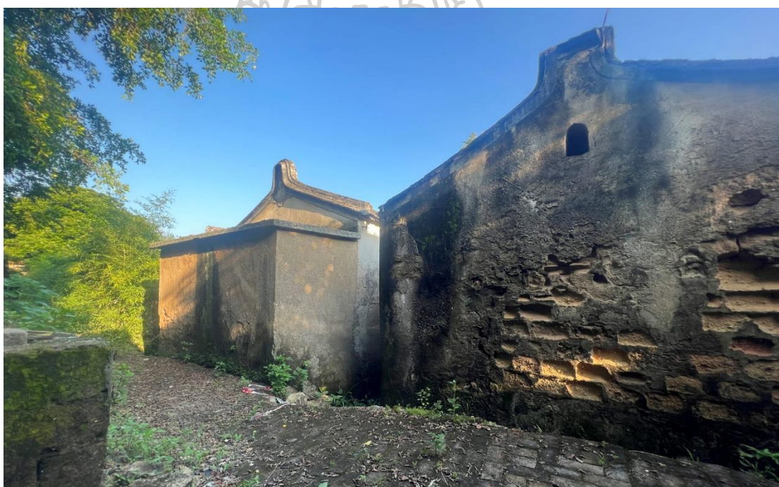
Figure 52. Moderately Damaged, Woshicun
