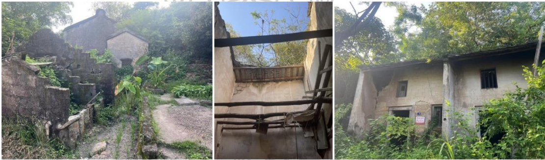
Figure 120. Damaged and Severely Damaged Buildings, Woshicun
