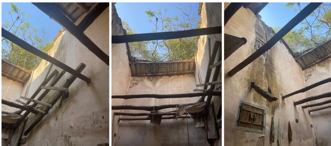
Figure 51. Severely Damaged, Woshicun
