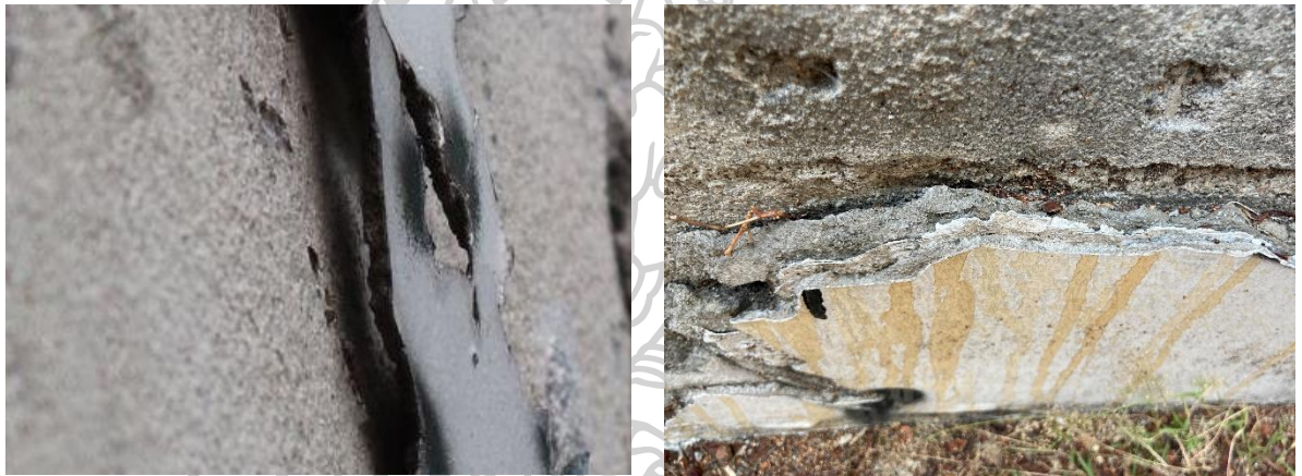
Figure 68 The loose part between the plaster layers Source: Elias Campidell (June 12, 2023)
