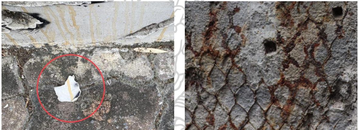
Figure 70 A fragments of the wall's plaster on the floor Source: Kawinthip Kittiphong (June 26, 2023)
