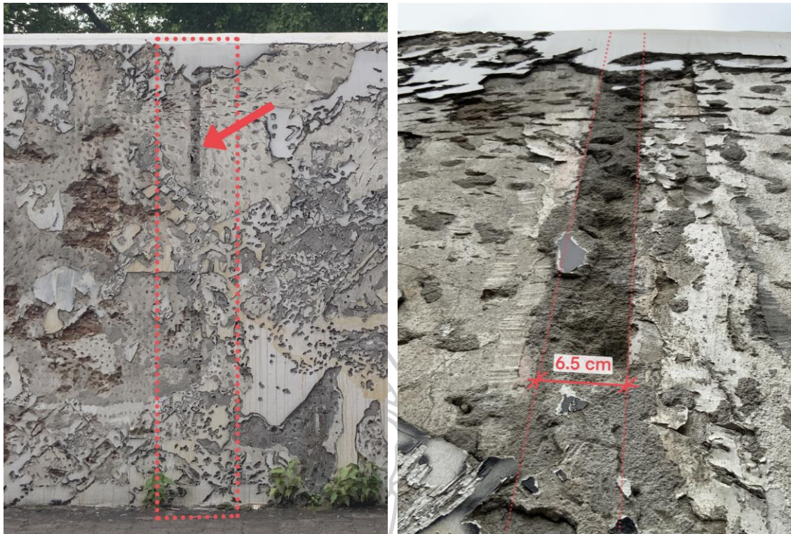
Figure 33 The position of a vertical support column in the wall Source: Khakhanang Jonganurak (August 9, 2023)
