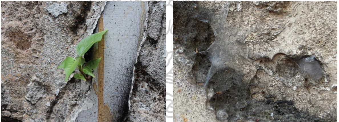
Figure 61 The growth of plants in the wall's crevices Source: Elias Campidell (June 12, 2023)
