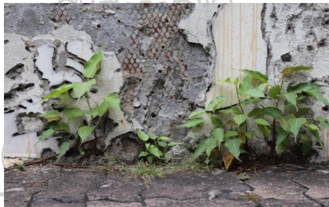
Figure 74 Plants and weeds growing in the lower areas of the wall Source: Elias Campidell (June 12, 2023)
