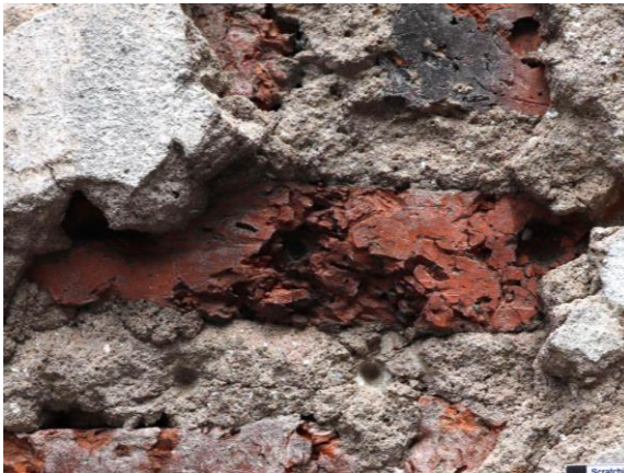
Figure 64 Cracking and crumbling brick Source: Khakhanang Jonganurak (June 12, 2023)
