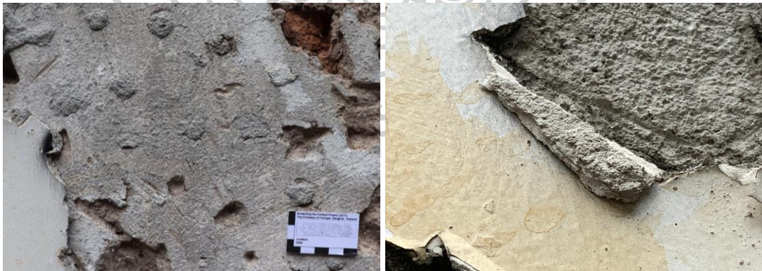
Figure 46 Traces of keying the plaster Source: Khakhanang Jonganurak (June 12, 2023)
