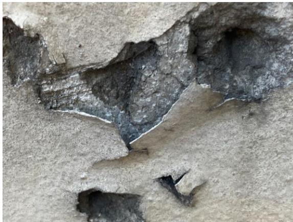
Figure 75 Peeling of paint layer Source: Khakhanang Jonganurak (June 12, 2023)
