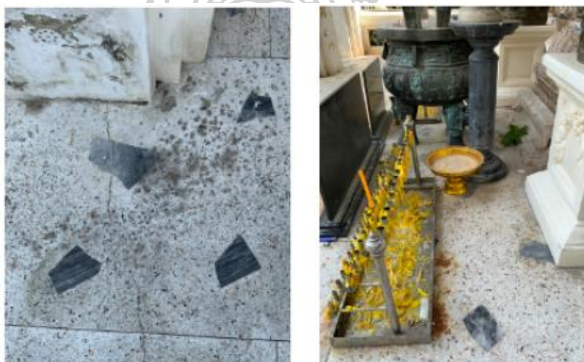
Cracked line on the terrazzo floor. Buddhist activities caused the floor's stain.
