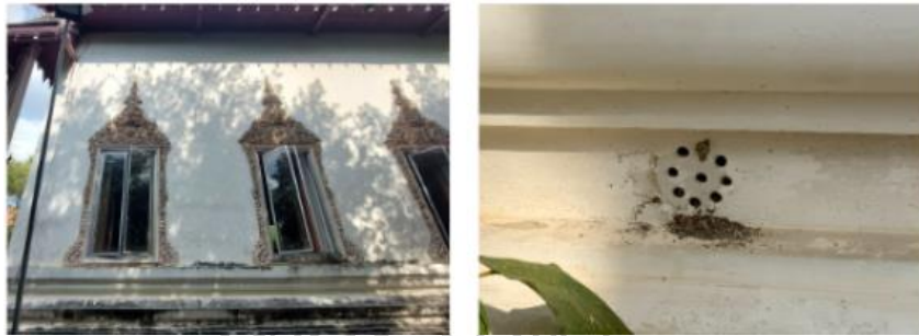
Deterioration on the wall of the ubosot . Ventilation hole round the exterior wall of the ubosot .
