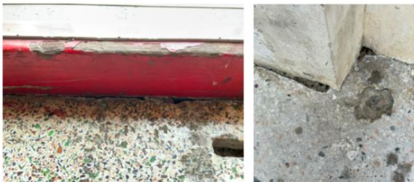
Deterioration of terrazzo floor and door frame. Deterioration of terrazzo floor.
