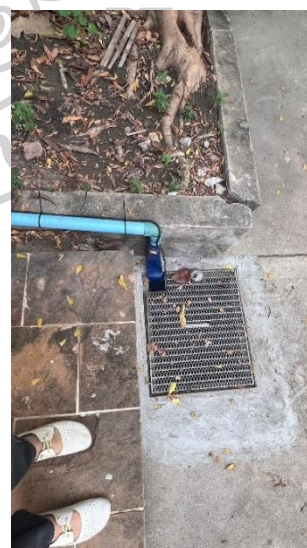
Fig. 36: Small holes for water collecting and drainage pump pipeline, Wat Kampang at Klong Bangjak canal. On 1 st April 2023.
