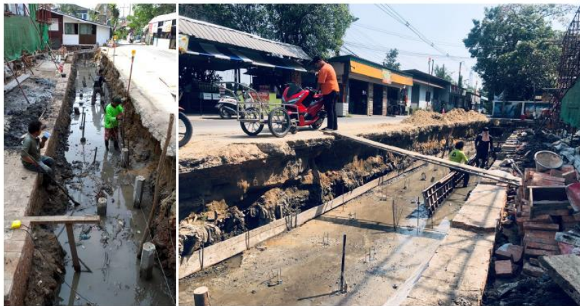
Fig. 16: When the foundation for the boundary fence was built, the underground water was shown.
