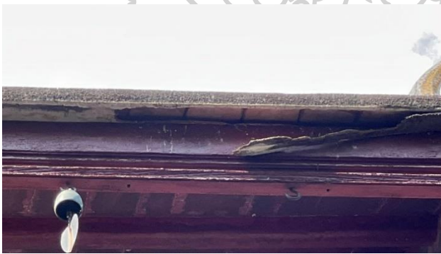
Fig. 78: The timber deterioration of the roof structure, Wat Kampang at Klong Bangjak canal. On 6 th February 2023.
