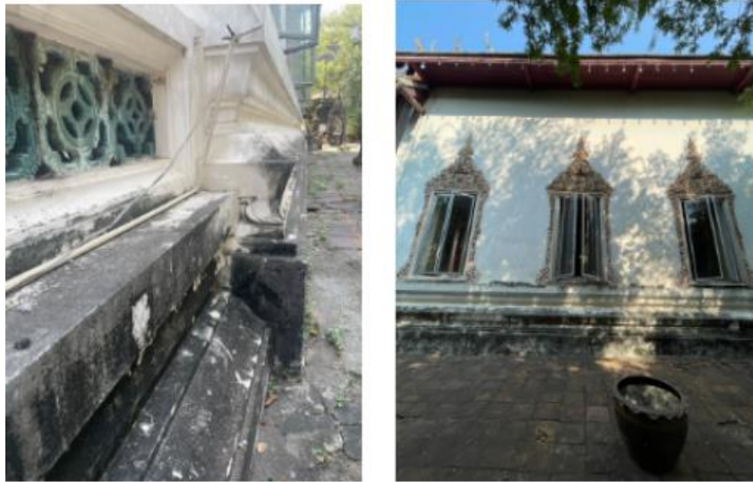
Deterioration on the base of the ubosot . Terracotta tiles and planting pot.
