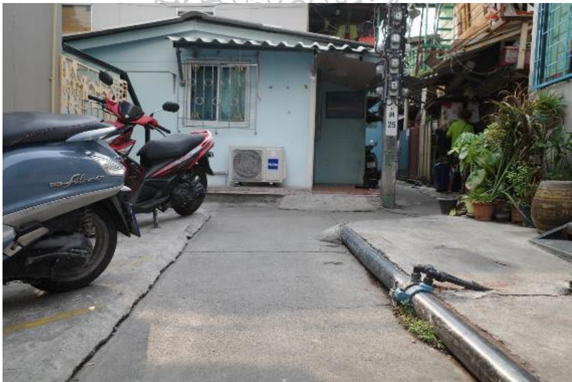
Figure 87 Micro elevation due to water pipes, etc.
