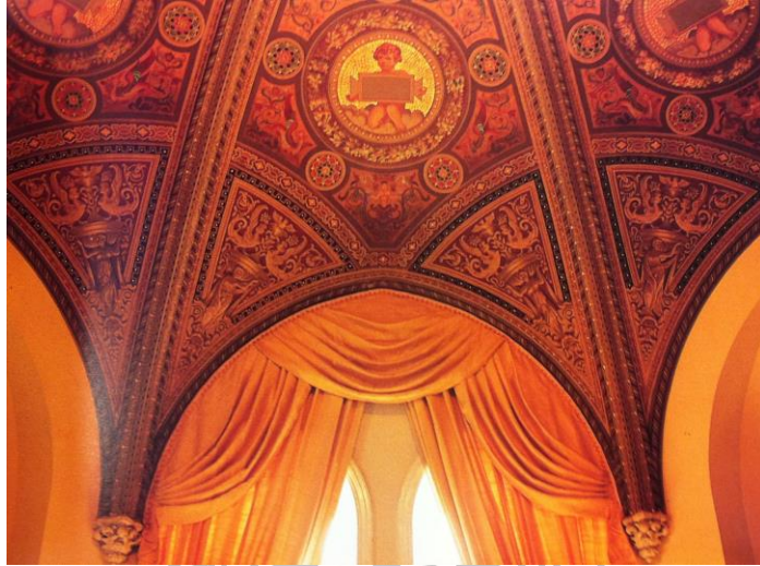
Figure 88 Villa Norasigh ceiling decoration (3) which fully western contents Source: Government House, The Royal Thai Government (Bangkok: Dansuttha Printing, 1987), 44.
