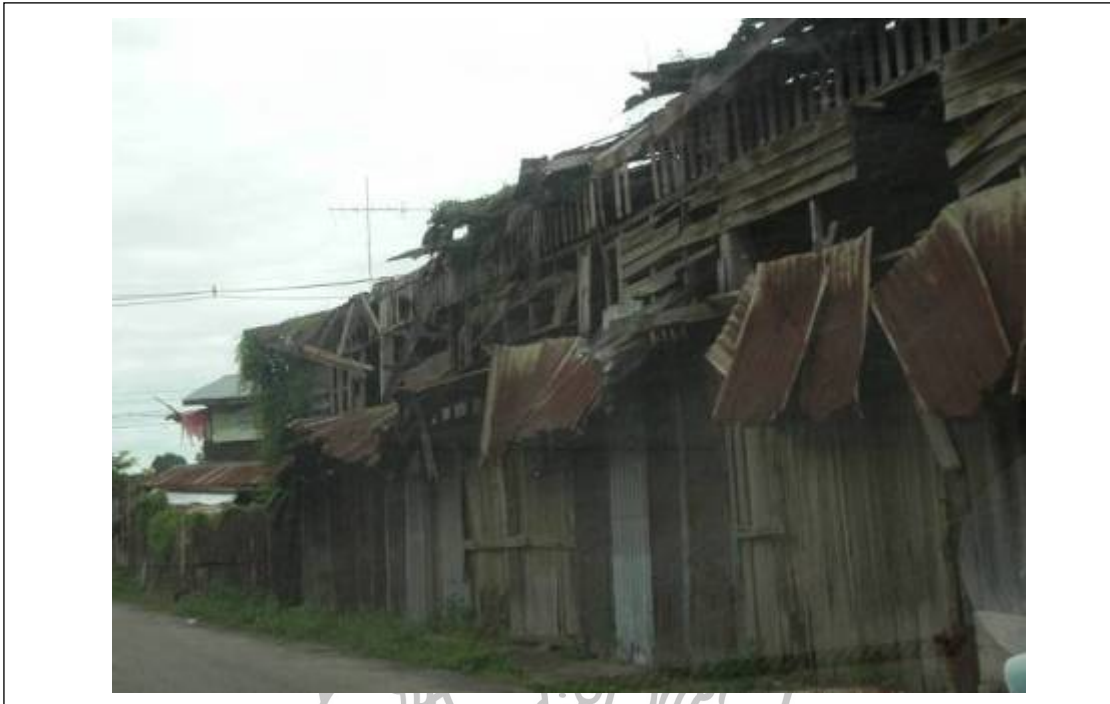
Figure 57 Abandoned row houses at Talad Lang
