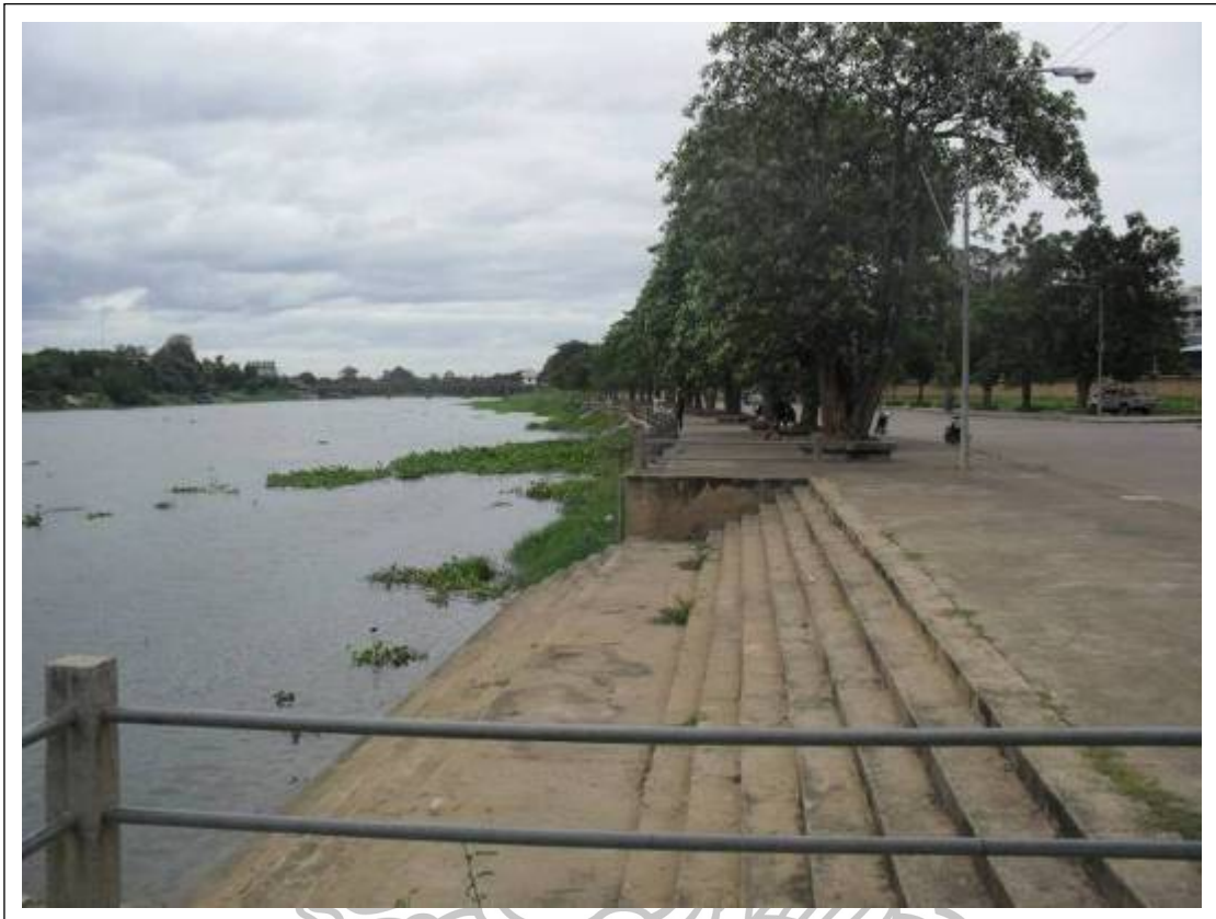
Figure 62 The concrete road parallel to the Maeklong river for countering soil erosion. Source: Author in June, 2012
